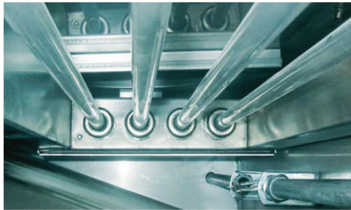
UV grease breakdown system within a kitchen canopy
