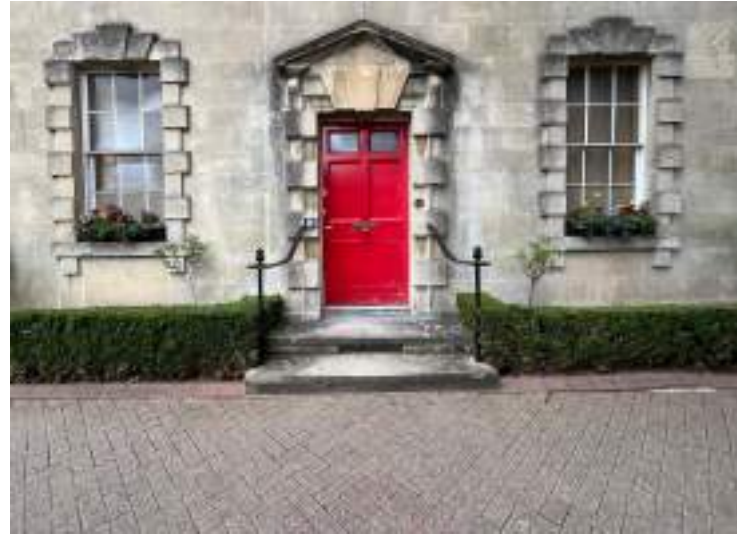
The existing condition of the front door, showing the paving design which dates from the 1980s.
