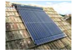
solar thermal panels for hot water
