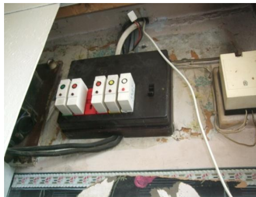
Fuse board, dated and no earthing
