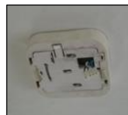
Disabled smoke alarm with the cover removed
