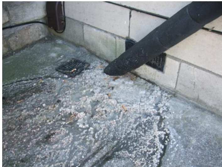
Blocked front drain
