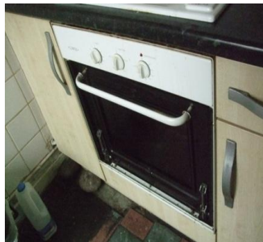
Front panel missing off oven
