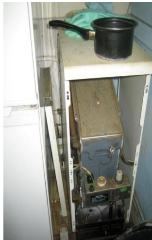
Damaged boiler with front panel missing
